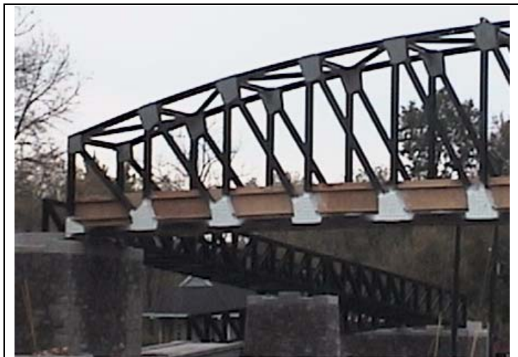
This pedestrian bridge was installed across Route One in the early morning hours of October 18 th . The bridge reconnects the towpath of the D&R canal for the first time since the early 1970's. A formal dedication and opening is expected in spring, 2004.
